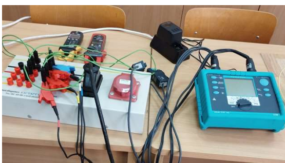
Fig. 4. General view of the connection diagram of power quality analyser for studying the electric power of induction motors.
