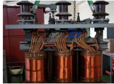
Fig. 5. Three-phase 500 kVA distribution transformer used in this study.
